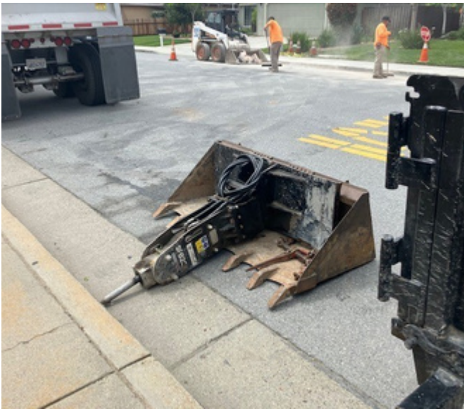
Encroachment Permit Violation
